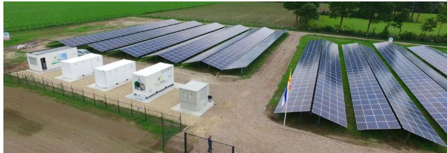
Energy storage at solar park Weert Energie
